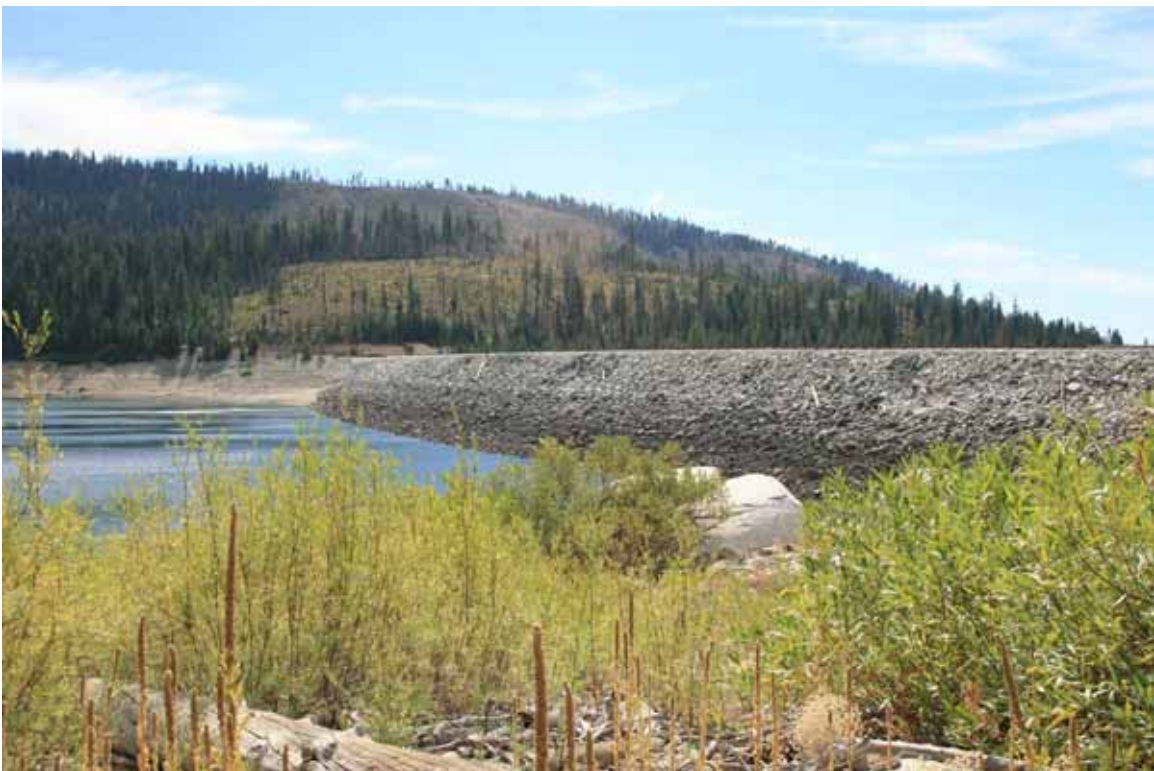
Photo 6. View of upstream side of French Meadows Dam from French Meadows Reservoir viewshed (near Spillway), looking south.
