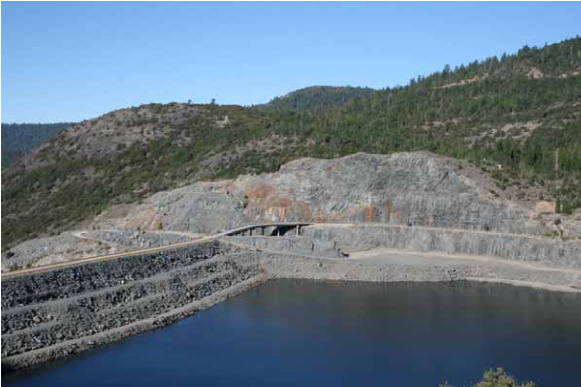
Photo 14. View of Hell Hole Dam and Spillway from Upper Hell Hole Trail (Hell Hole Reservoir viewshed).
